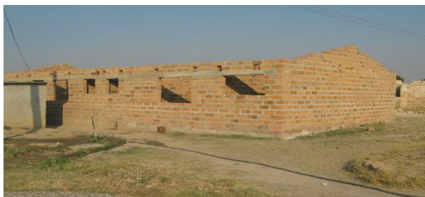
Figure Error! No text of specified style in document.-3 source: field work pictures
