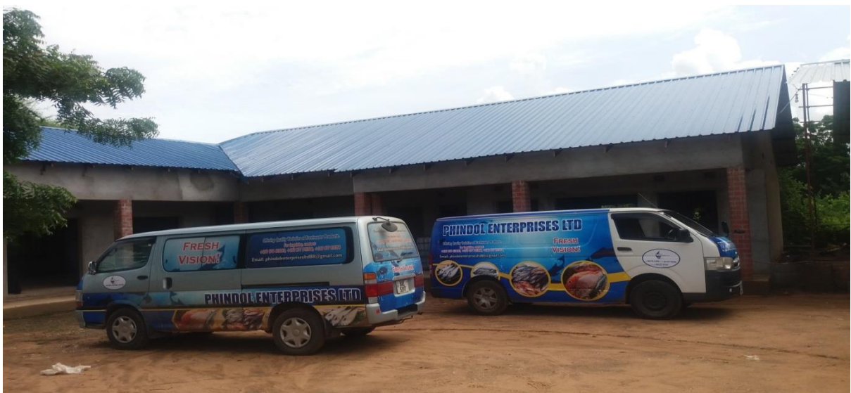
PEL 2. This picture shows the new offices of PEL under construction with some utility vehicles
